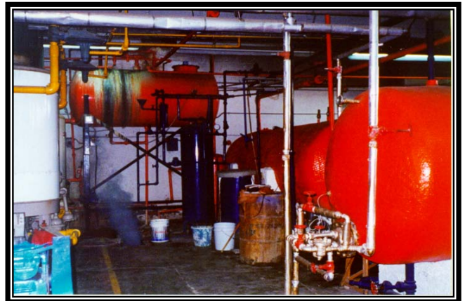
Old Steam Generators and Hot Water Tanks
