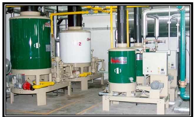
New Presence of the boiler room
