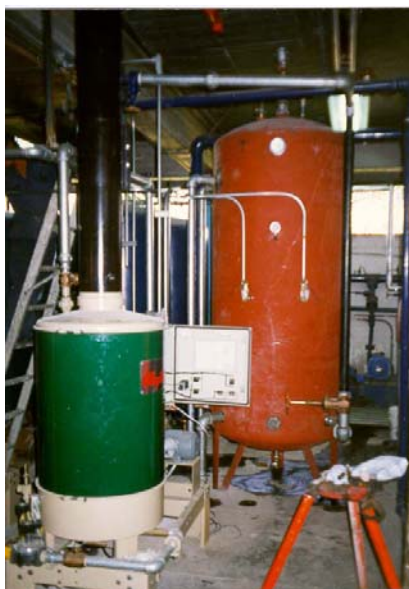
Small tank for direct hot water recirculation
