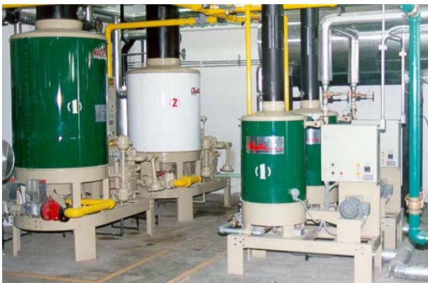
New Presence of the boiler room
