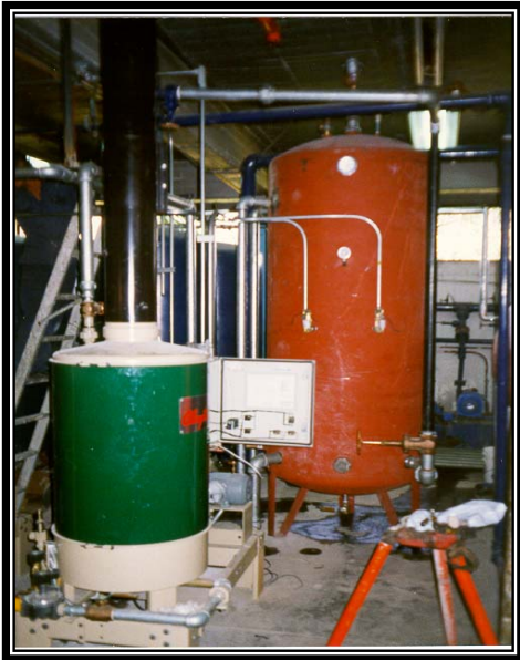
Small tank for direct hot water recirculation
