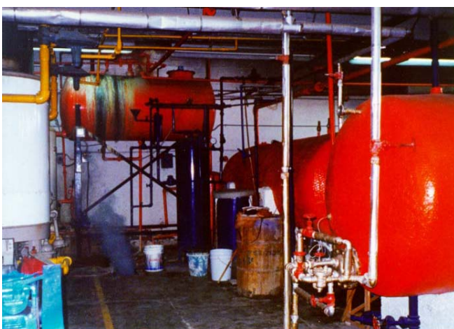
Old Steam Generators and Hot Water Tanks
